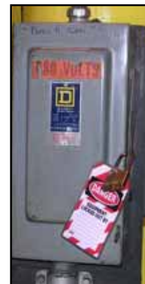
Figure 2: Lockout/Tagout on the Power Source Panel
